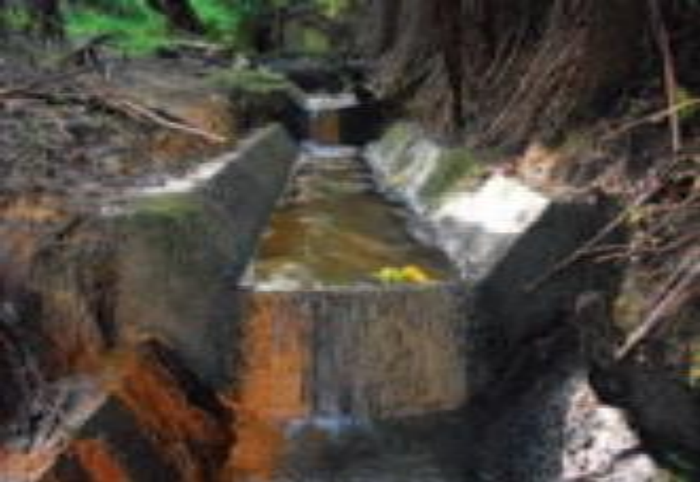
Partial barrier - swimming species unable to pass
