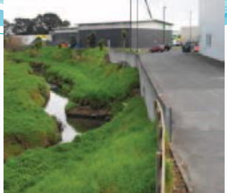
Floodplain connectivity restricted by development
